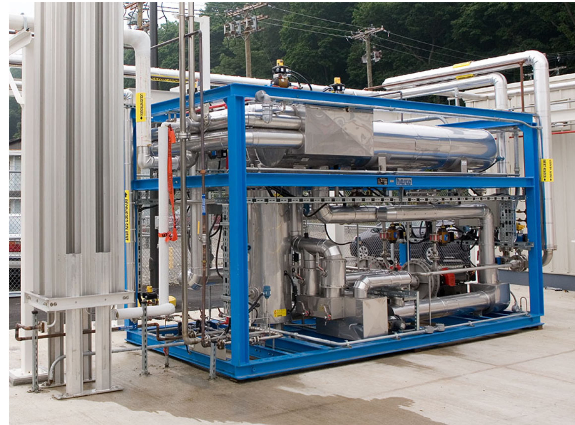
Vertical Dryer & Condenser for Separating Electrolyte
